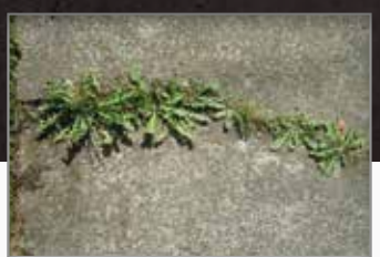
Weeds on pavement
